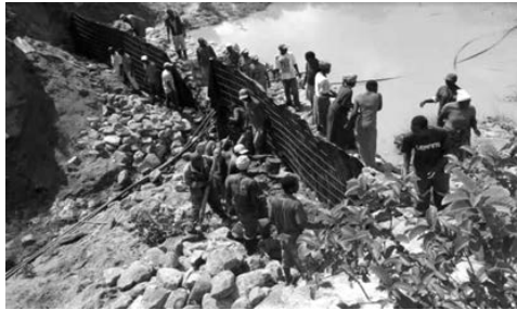
The Manyenga dam, in Mutoko District. Part of the BRAC programme, which is helping communities adapt to climate and socio-economic shocks in Zimbabwe. Photo: Christian Aid
